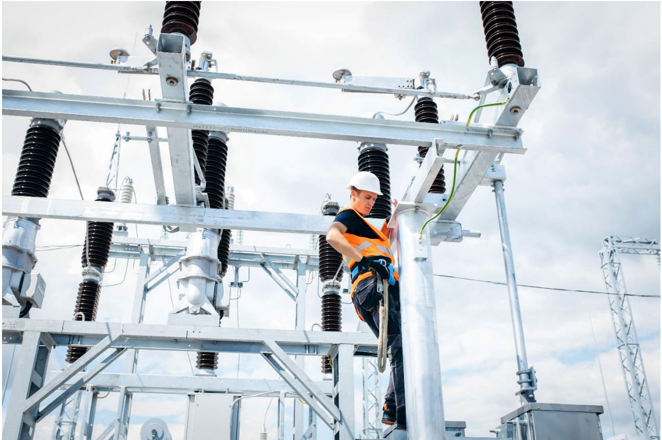
An electrician services a high-capacity transmission station.
