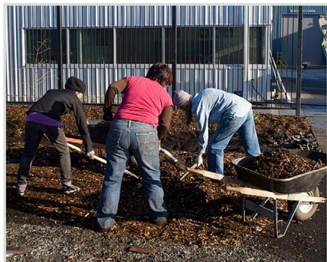
The Georgetown Community Council, working with the nonprofit Duwamish River Cleanup Coalition, helped lead the construction of stormwater swales.
